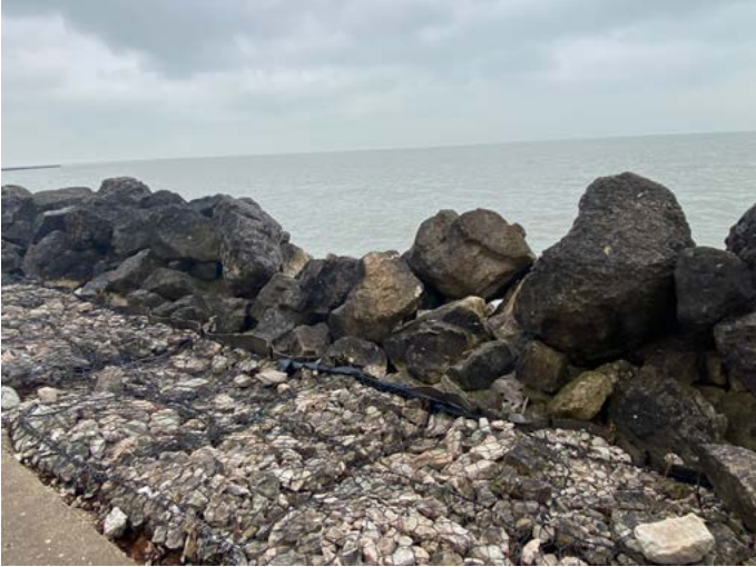
Image 2: Section loss in revetment crest
