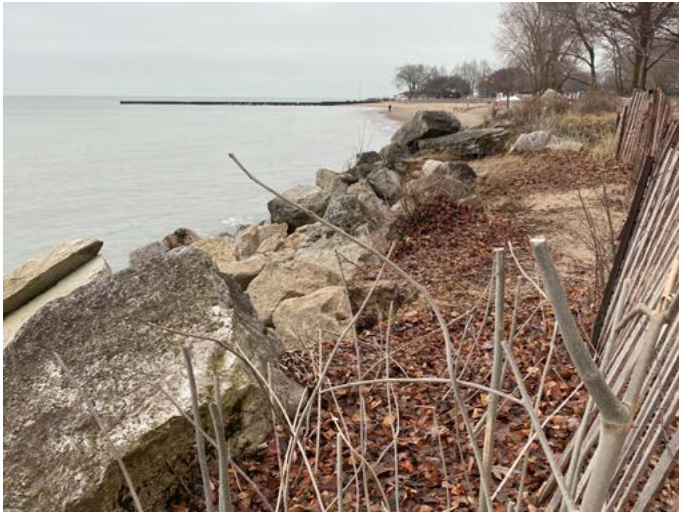
Image 1: No significant revetment crest
