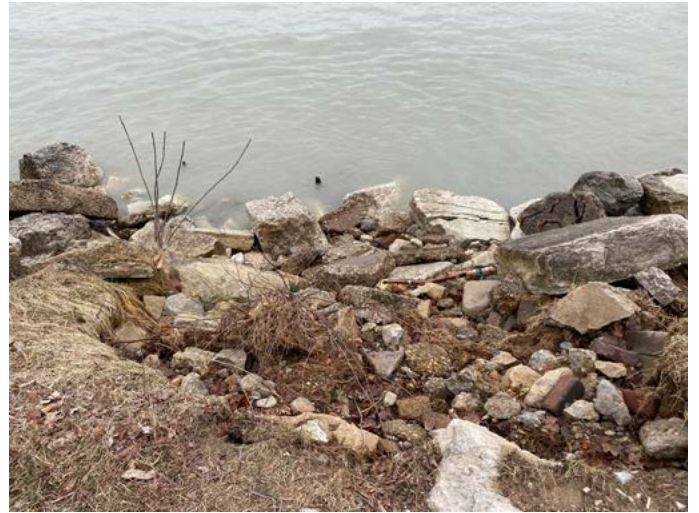
Image 2: Section loss and exposed underlayer
