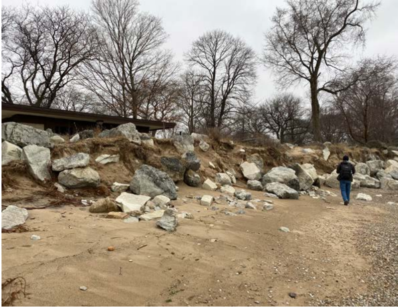
Figure 1-1 Erosion at Greenwood Beach (March 2020)
