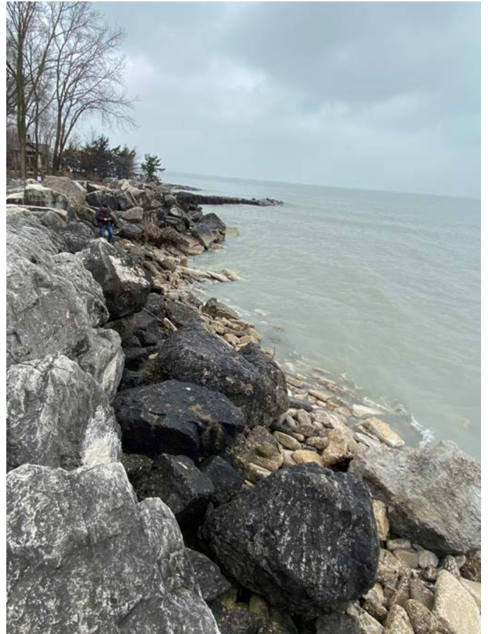
Image 2: Exposed underlayer and section loss throughout revetment
