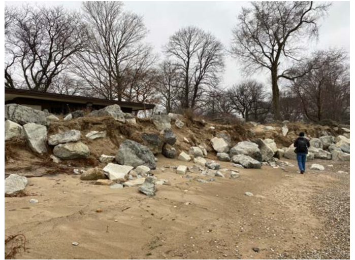
Image 2: Large slope failure with scattered stone
