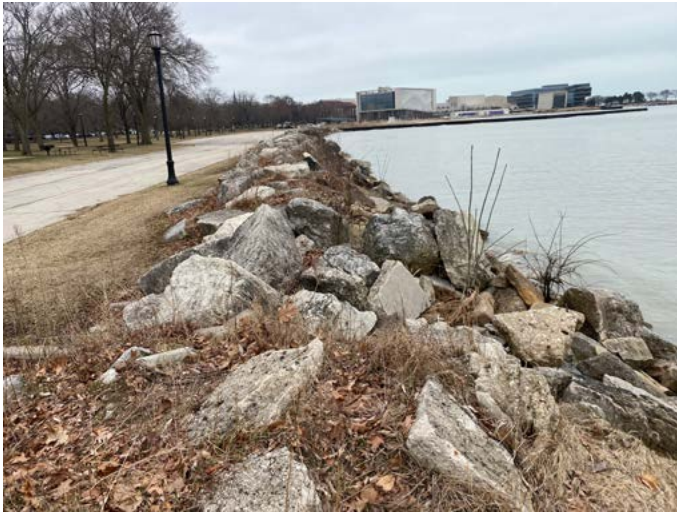
Image 1: Variable amount of stone at revetment crest
