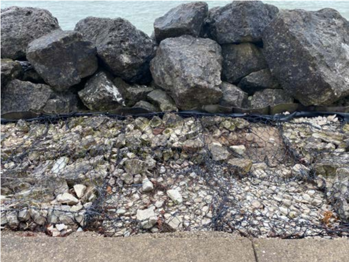
Image 3: Damaged gabions on back side of sheet pile wall
