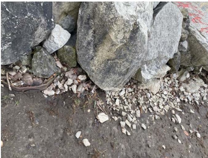
Image 3: Erosion and exposed sheet pile wall at back of revetment
